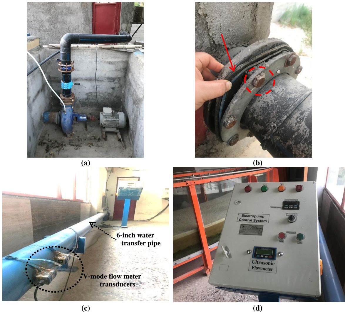
Figure 2. Installation of the pump and the flowmeter: (a) the installed pump, (b) 1- the waterproof rubber O-ring sealing gasket, and 2- bolts and nuts, (c) the flowmeter transducers in V-mode, and (d) the flowmeter control box
