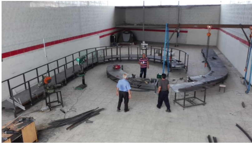
Figure 4. Construction of the structure and assembly of the first channel in Azar Ashena Ab Co
